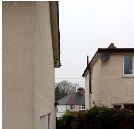
Image 3 - Photo of side elevation from rear of 48A (left) and no.48 (right).
